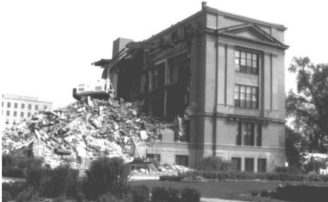
Fig. 2. August 12, 1993, the Wisconsin High School is demolished to make way for the Biotechnology Center. [Author Photo, AP-9]
