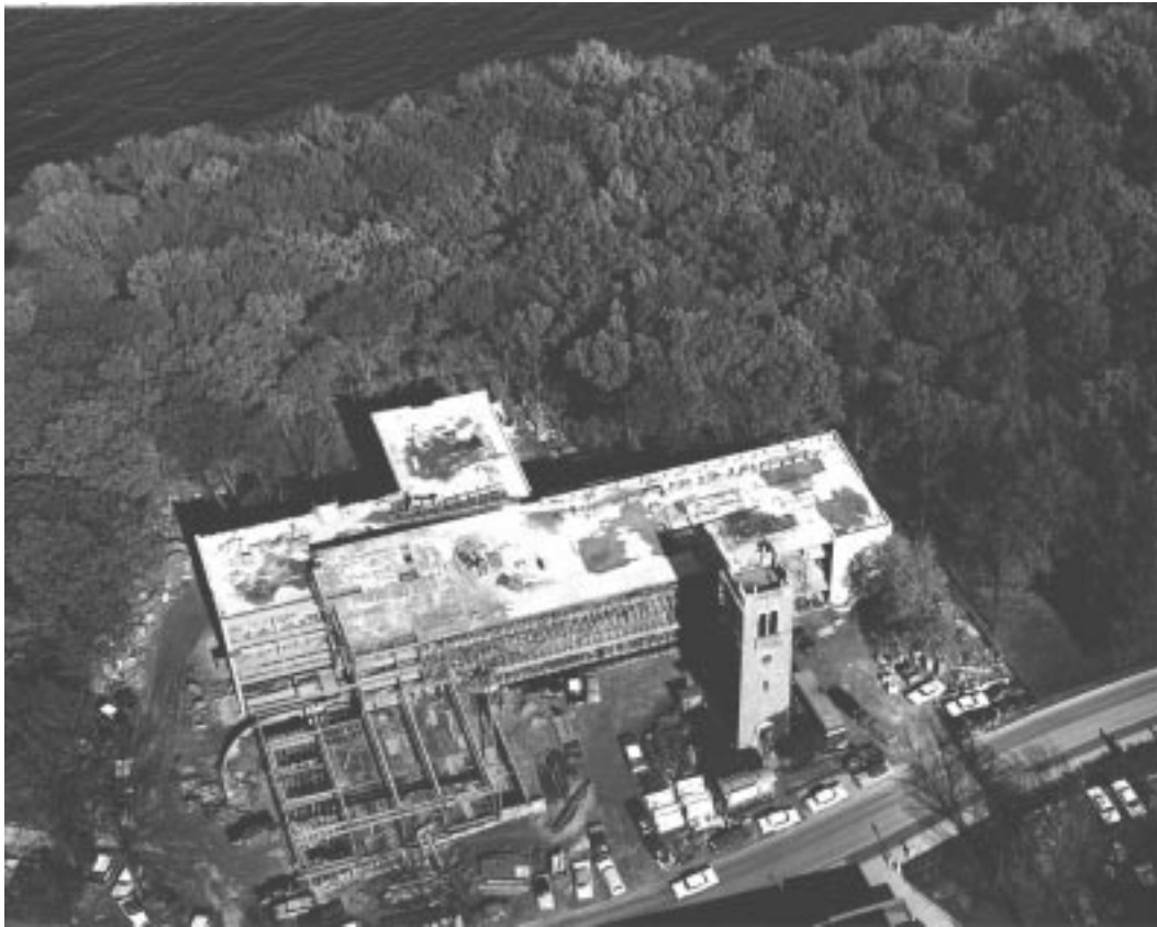
Fig. 2. October 27, 1961. Social Science under construction. Note the density of the wooded area to be developed to the north of the building. This is the Bascom woods that was so heavily defended by the Capital Times and others. [Series 9/1, Social Science, ns-2949]
