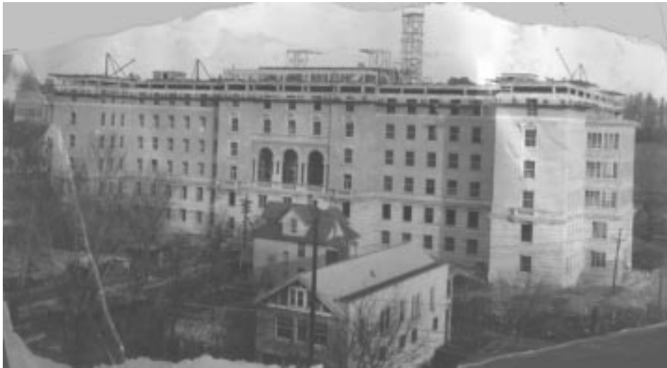
Fig. 2. Wisconsin General Hospital under construction from University Avenue, c. 1923. [Meuer photo, vol. 10, p. 69]
