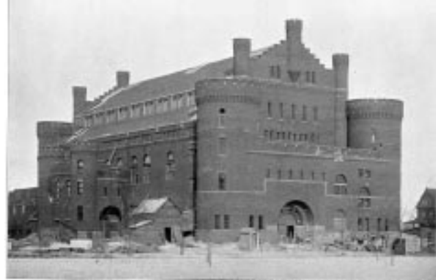
Fig. 2. Gym during construction 1894. Sheds in foreground held temporary boiler and tools. [Armory/gym folder #1 jf-21]
