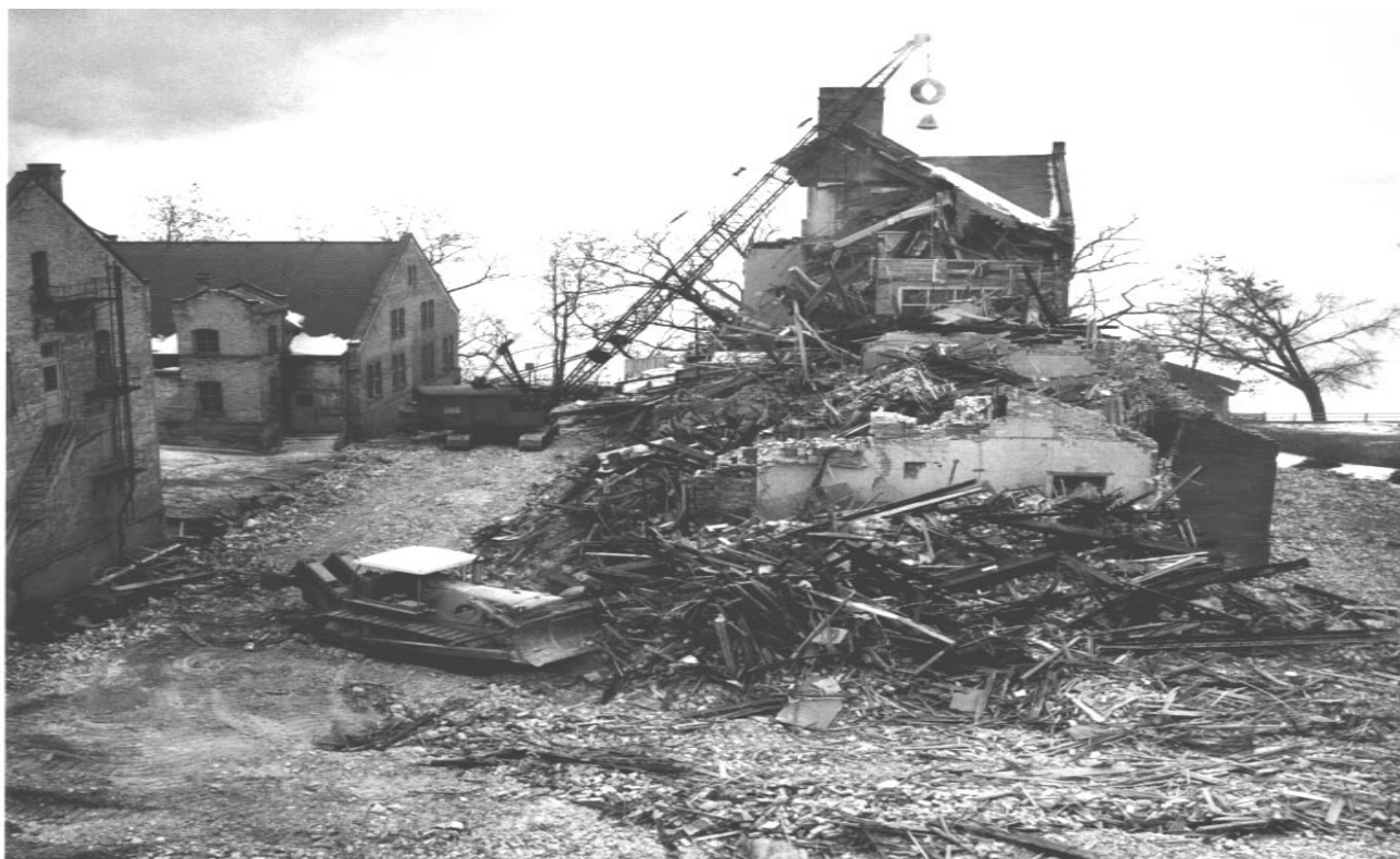
Fig. 3. The first chemistry building comes down in 1965 to make way for Helen C. White Hall. The machine shops are on the left; they were demolished next. [Helen C. White folder ns-3110]
