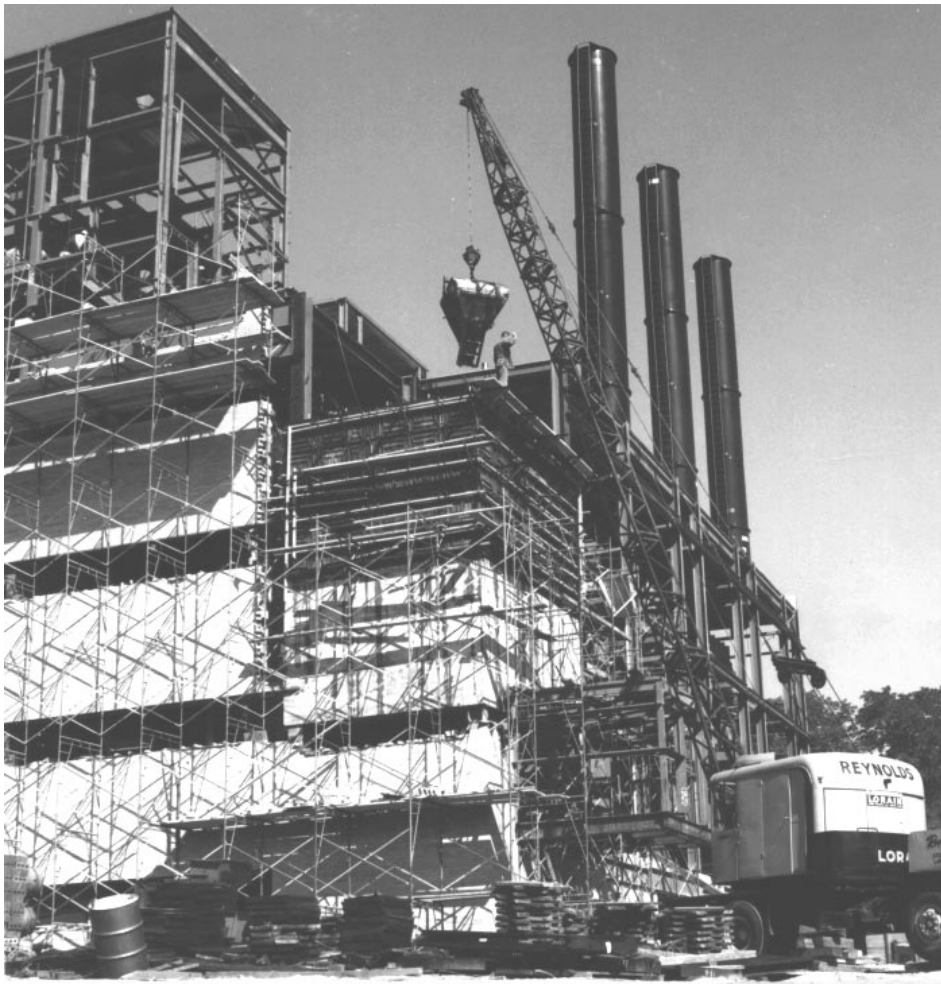
Fig 2. The erection of the American Motors heating plant, summer 1958. [series 7/4 folder #2, jf-99].
