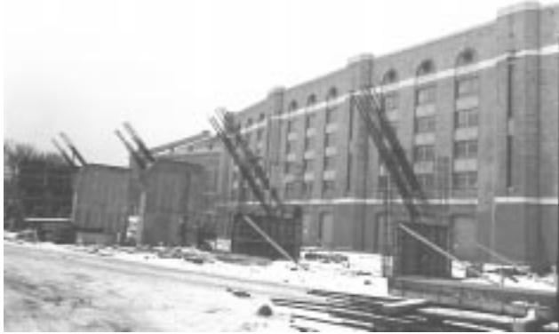
Fig. 2. The Camp Randall Shell under construction, 1954. The stadium domes are in the background. [series 9/10/3, ns-256]
