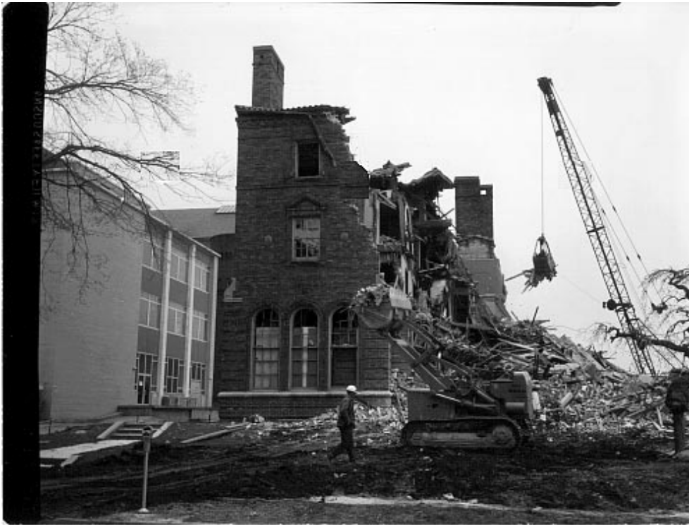
Fig. 2. The demolition of the Sigma Chi fraternity house April 24, 1965. The site of the new alumni house.
